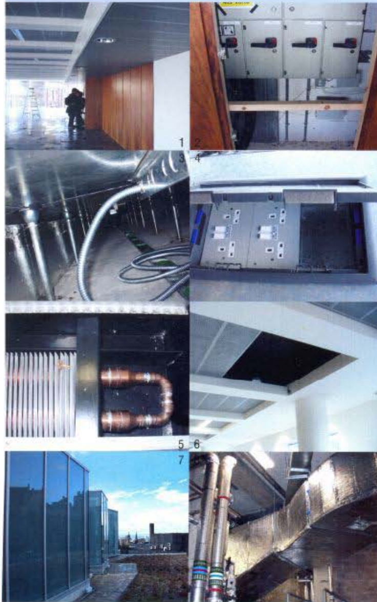
Fig 2 How the services strategy integrates efficient service distribution, daylighting, circulation, ancillary accommodation, structural concept and historical typology.
